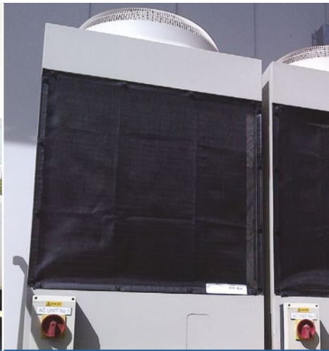
Chillers, dry air coolers & air conditioning units
