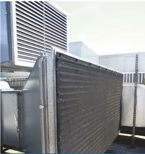
Air Handling Units
