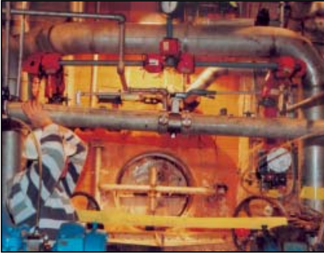
For externally corrosive environments, Victaulic offers a full line of stainless steel couplings, valves and fittings. The Series 763 butterfly valve on this line has been joined to the system using two stainless steel rigid couplings that match the performance and hanging requirements of welded systems.
