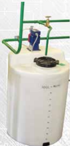
Chemical Dosing Set
